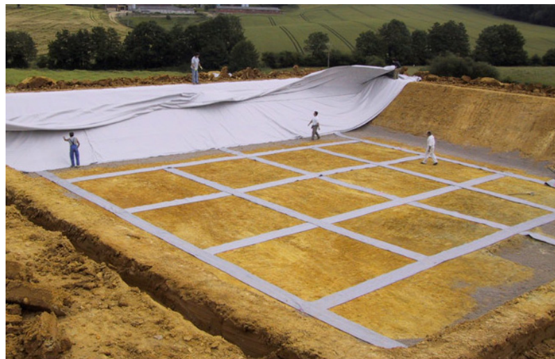
Photo : Gas drainage at the bottom of the basin (Wavin, 2014)
